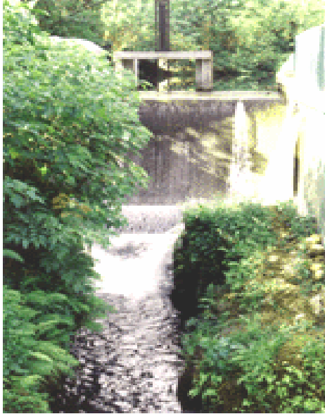
A view of the microhydro plant at Villa Escudero Plantations and Resorts, Inc., Philippines, Villa Escudero
