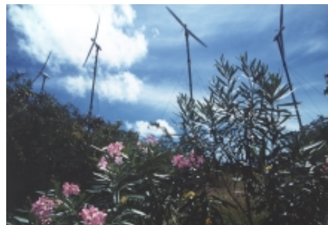
Four 60 kW VERGNET wind turbines on Marie Galante Island, Guadeloupe, French West Indies, ADEME
