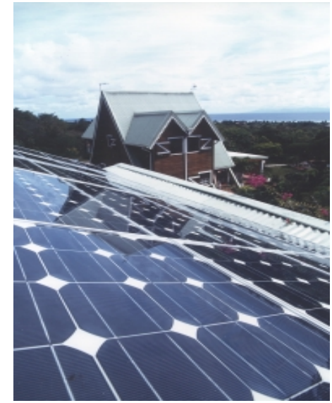
Photovoltaic installation on Marie Galante Island, Guadeloupe, French West Indies, ADEME
